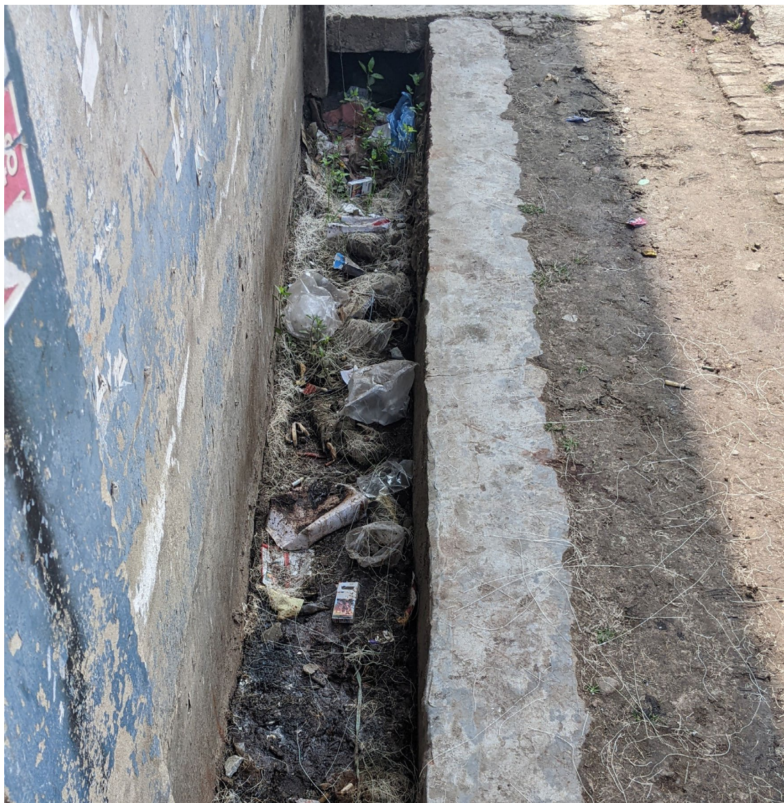
Figure 1: Drainage system clogged by plastic waste. Tanvir Ahmed, 2024.
